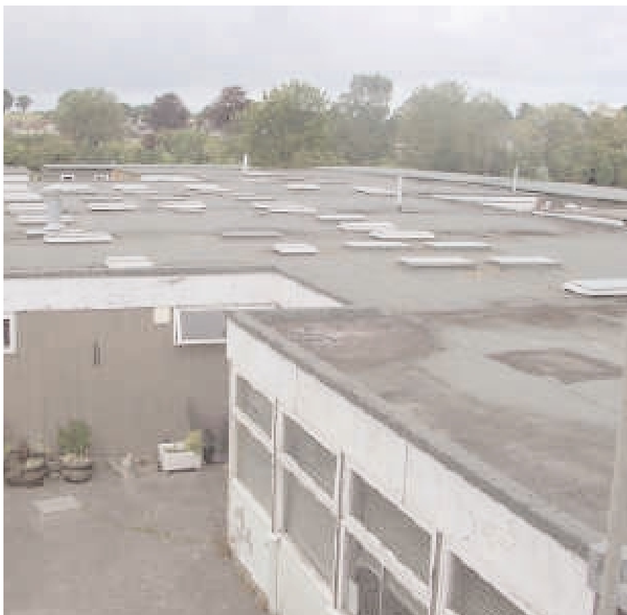
Figure 8 Allenbourn School's web page picture, captioned 'The current school – now you can see why we're getting a new one!!' ( www.allenbourn.dorset.sch.uk/Buildings home page.htm )
