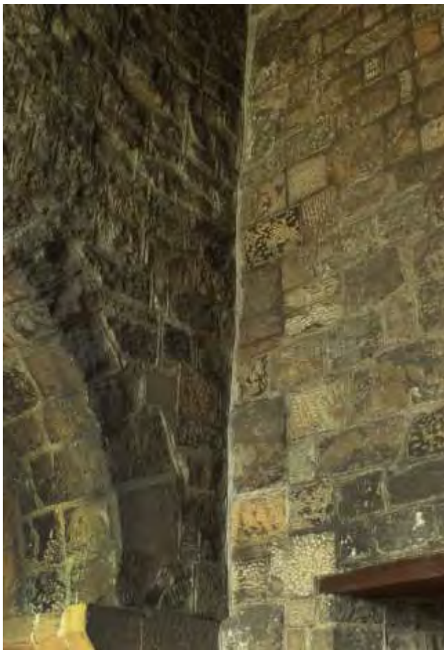
Figure 7b: North western interior corner of the Eastern Church, showing sheared quoins.
