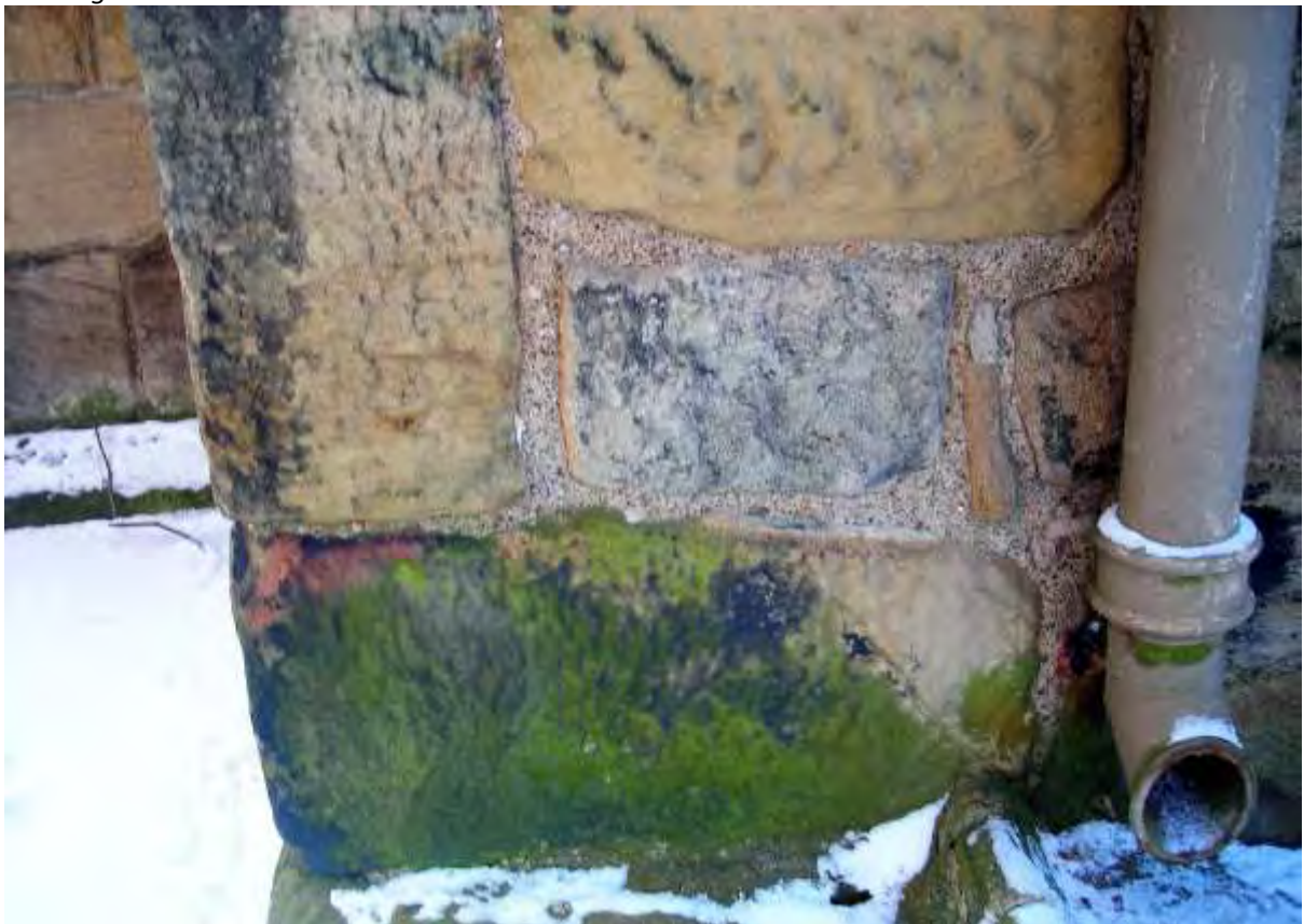
Figure 15: One example of several quoins at both churches, whose shape resembles modified Roman altar stones. This lies at the external south-east corner of the east end St. Paul's, Jarrow.
