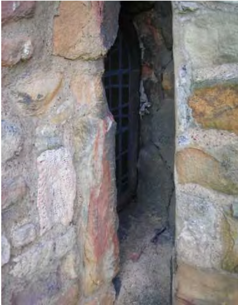
Figure 41b: Fire damage evident on the interior stonework in the western end of the nave at St. Peter's, Wearmouth.
