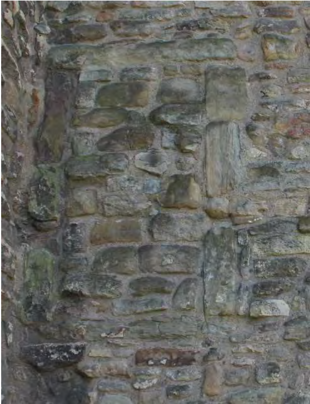
Figure 6: Infilled door with frame on north side of porch/tower, executed in soft sandstone from North Hylton
