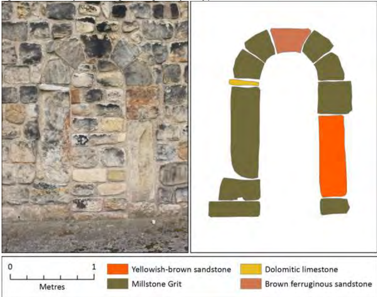
Figure 13: Roman stonework evident in the surround of the blocked doorway on the north side of the Eastern Church at Jarrow.
