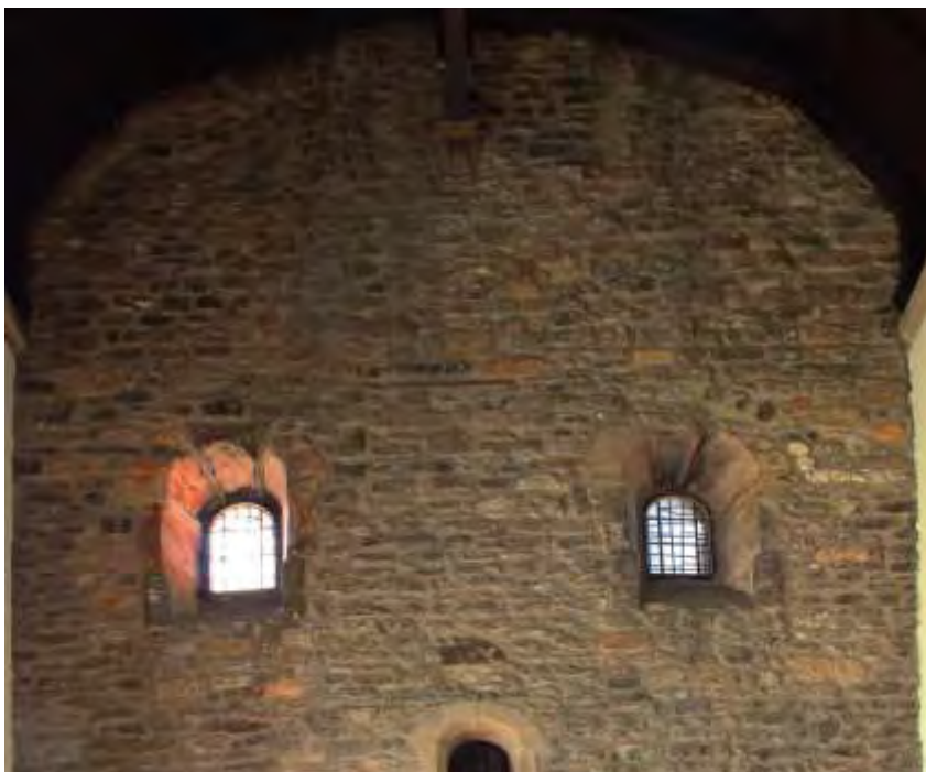
Figure 41a: interior stone work at the western end of the nave at St Peter's, Wearmouth, showing the burnt areas around the upper windows.
